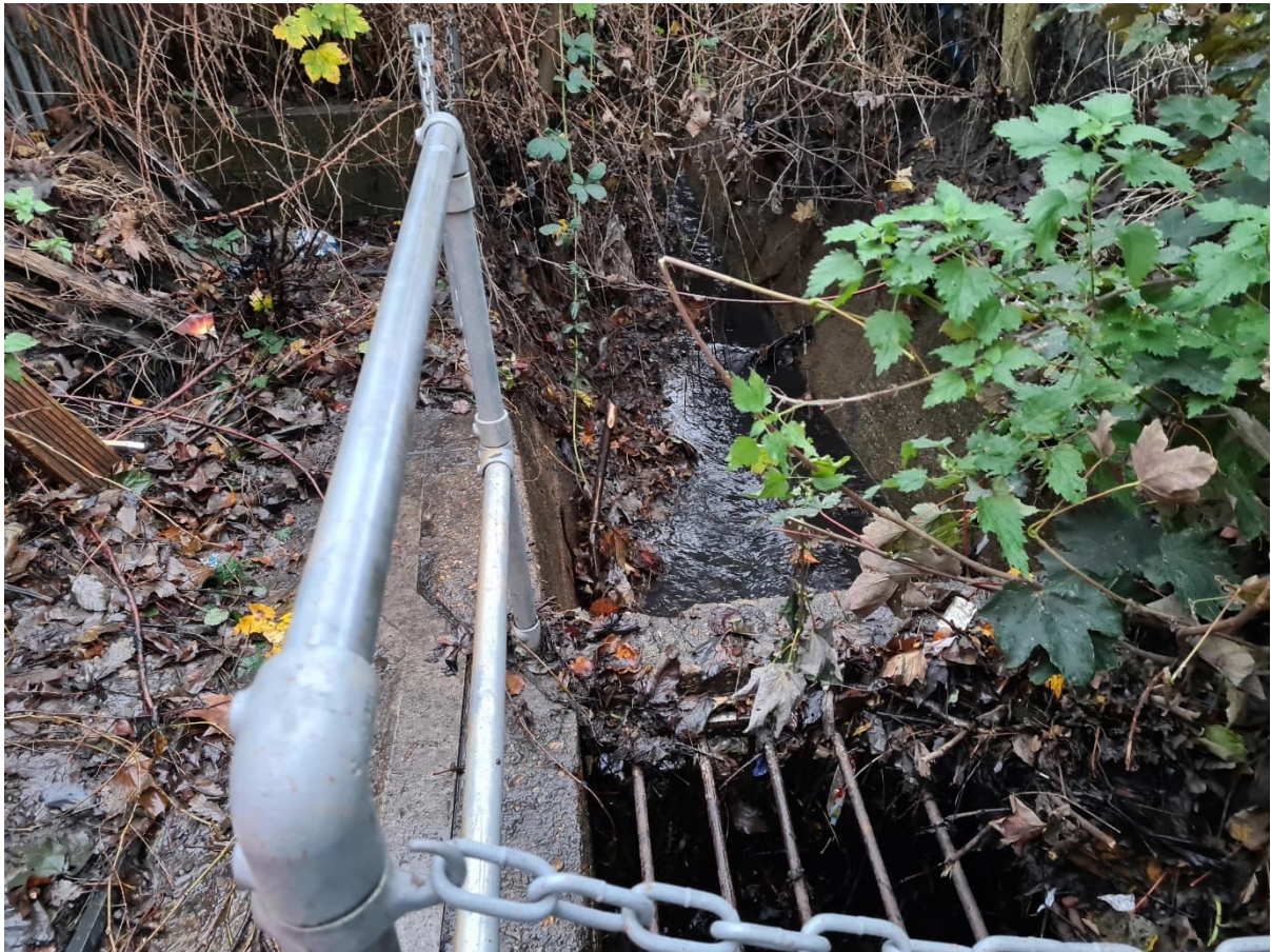
Photograph 4 Post screen clearance (07.11.2022)
