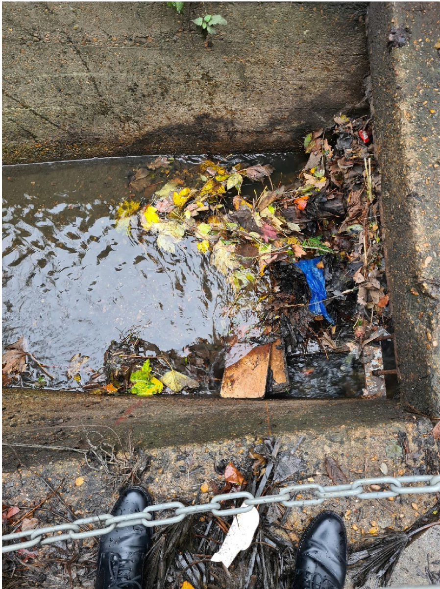
Photograph 5 Debris build up on the screen (29.11.2022)
