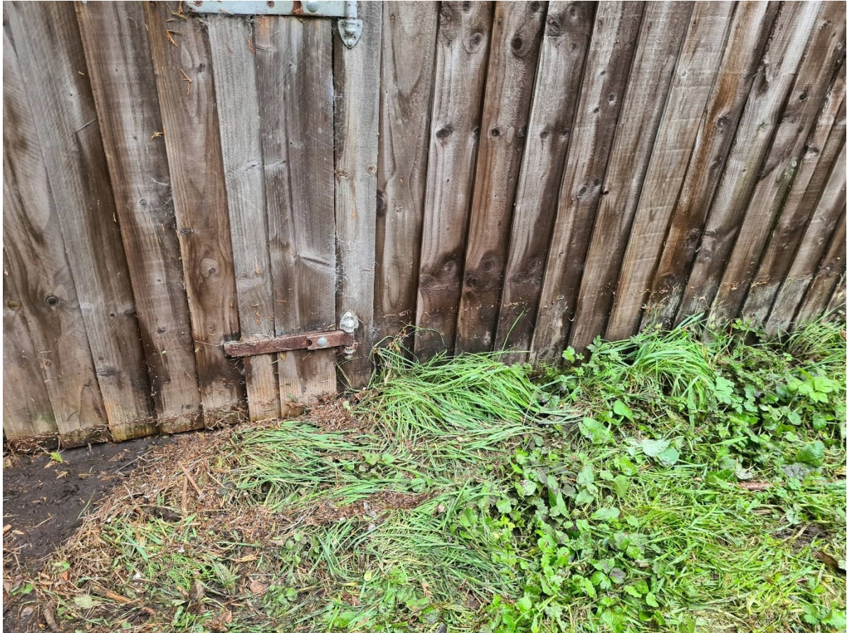
Photograph 1 Water level approximately 300 mm from ground level, reported by RBG (07.11.2022)
