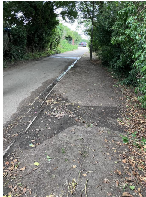
Photograph 7: Silted drainage channel along King John's Walk
