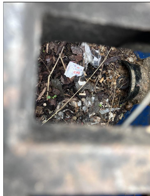
Photograph 14: Debris blocking a gully on White Hart Road.
